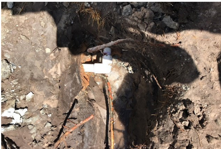
Figure 6 – Burst PVC Irrigation Pipe Elbow
