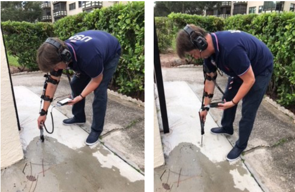
Figure 4 – Using the Sonaphone Ultrasound Tester to Pinpoint the Leak
