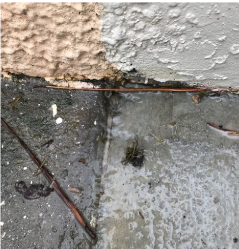
Figure 2 – Water Seepage Observed at the Site
