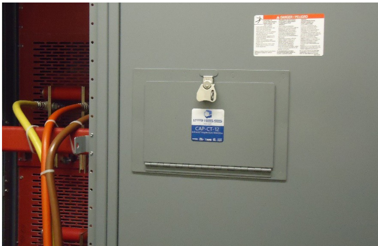
Figure 2 First Panel fitted with an IR Window
